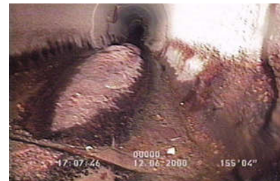
Debris build up
