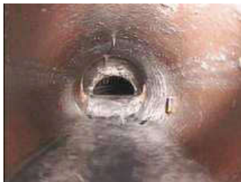
Partially blocked drain
