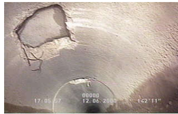
Severe damage to concrete pipe
