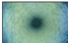
Boiler Tube - Pitting
