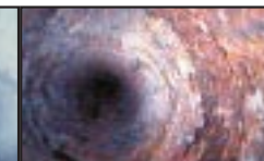
Drain Line - Corrosion
