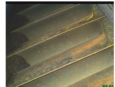
Turbine Blade Mineral Deposits
