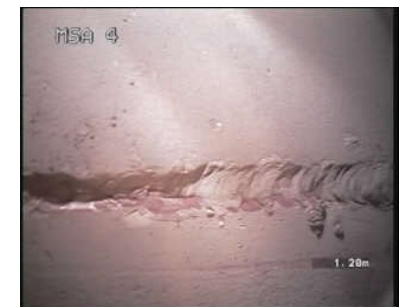
CMV Weld Crack
