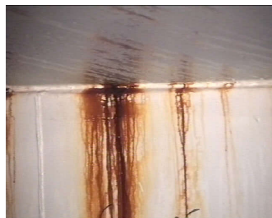
DeMin Tank Rust
