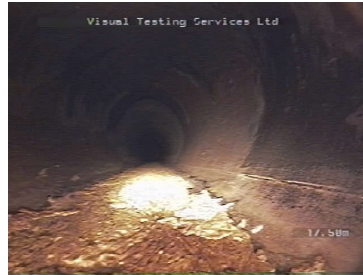
Debris in Flare Line
