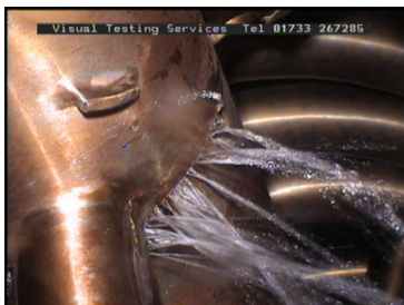
Heating Coil Leak
