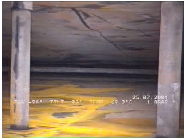
Tank Roof Distorted
